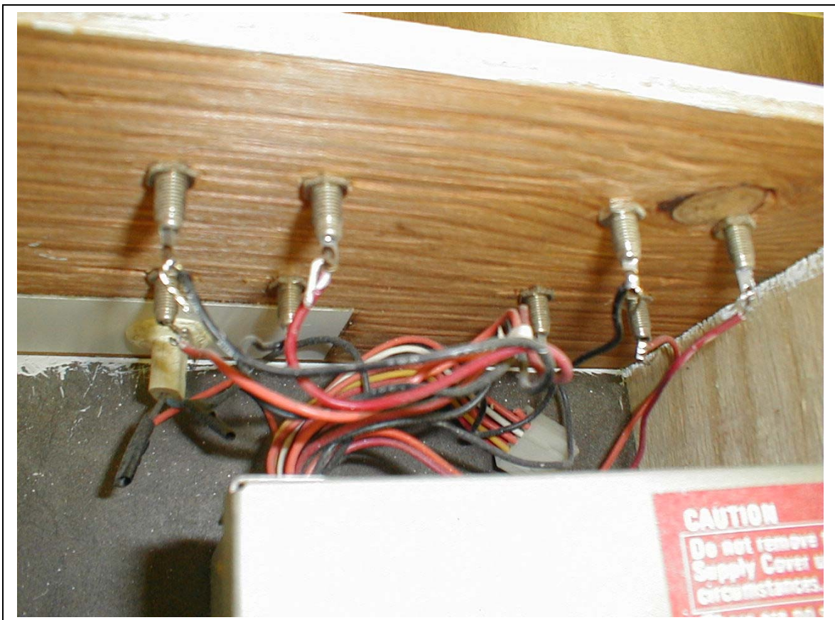
Figure 1B: Computer Power Supply (Inside Front Panel)
