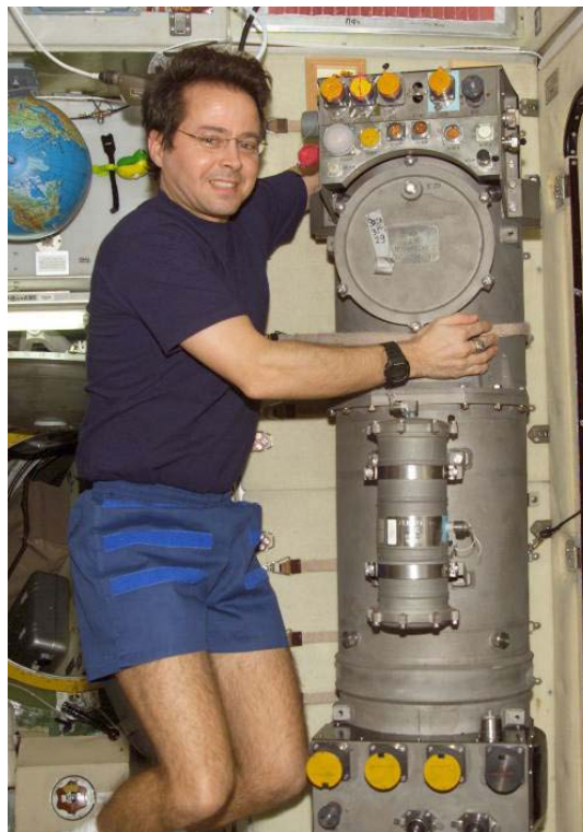
Figure 3: Astronaut Daniel W. Bursch working on the Elektron Oxygen Generator in the Zvezda Service Module on the ISS
